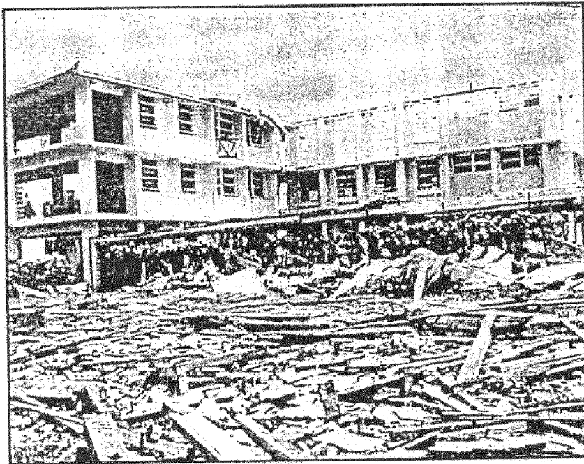
Figure 1. Hospital in the Caribbean severely damaged following a hurricane (Photograph: Tony Gibbs).
